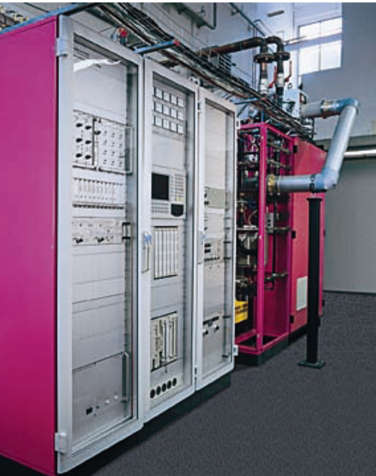
FIG 1 Control cabinet of 75 kW RF Amplifier VD741K1 (not including collector power supply) Photo 43 020
